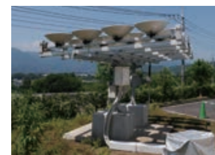
Tracking concentrator solar power generation system
